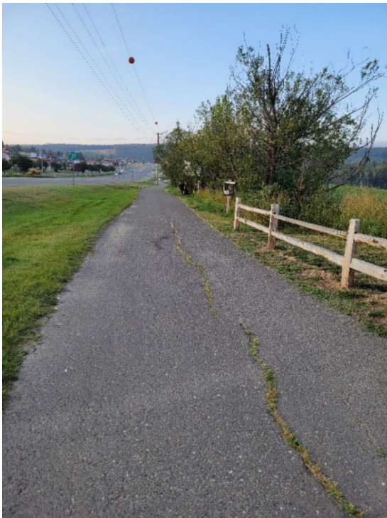
Marsh Trail – Poor asphalt condition may be difficult for some users.
